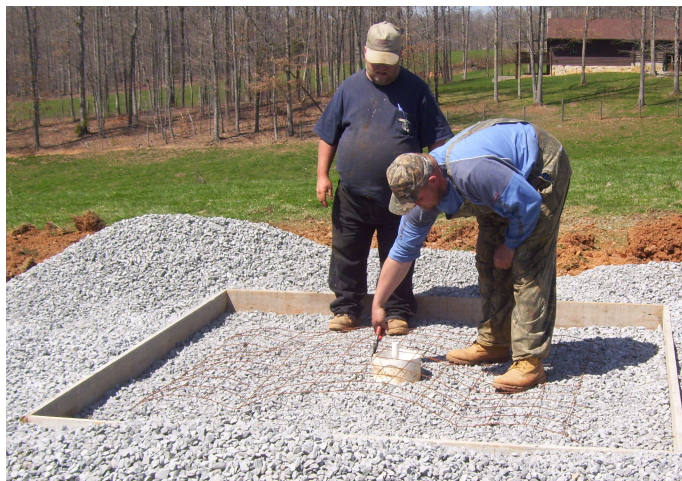
The anchor pad is installed to provide a level mounting surface for the trough. Earth tube is shown here being measured.
